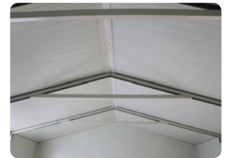
Strong Metal Roof Truss & Columns
