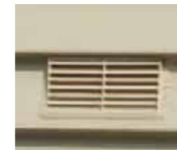
Air Vent for Ventilation
