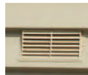
Air Vent for Ventilation
